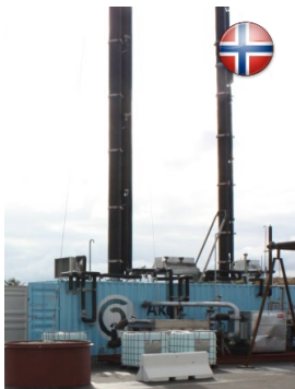
Natural gas Risavika Gas Center
